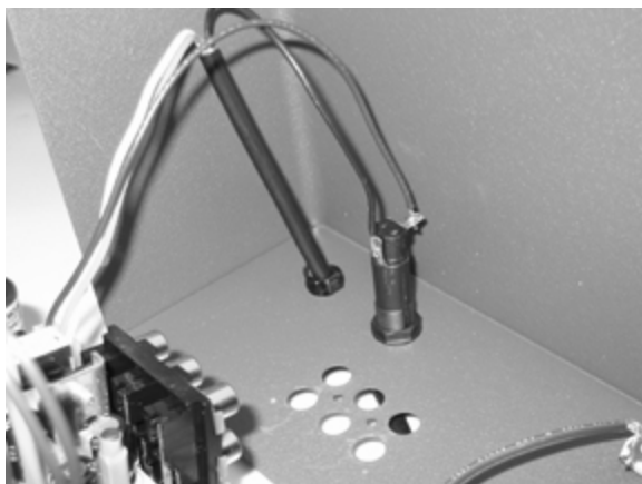
Fuse Wiring Close-up
